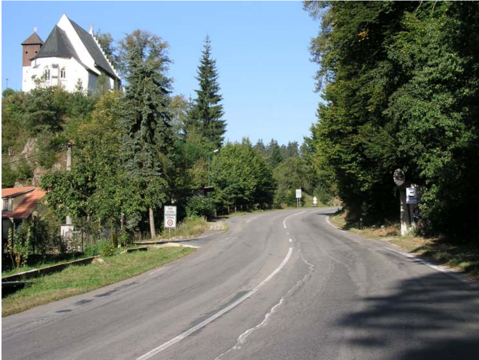
Svatá Kateřina – the state of the road and road marking is apparently poor.
