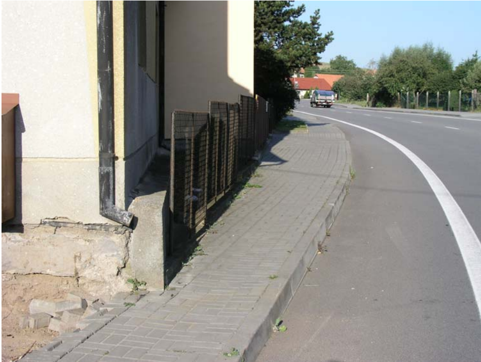
Narrow pavement in Šebrov – one can imagine that the pram cannot go through without entering the road.
